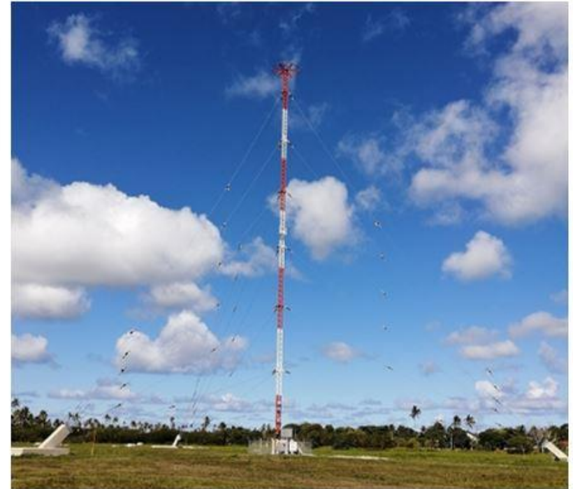
MW Antenna Mast
